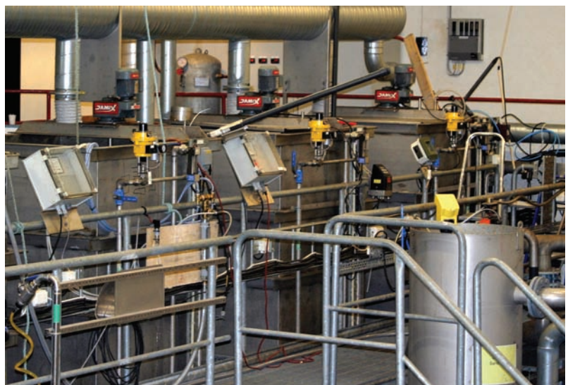
The test facility at the wastewater treatment plant at Hammarby Sjöstad.
