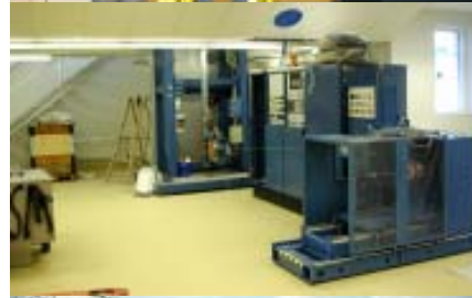
Control equipment of drawing tower middle of May
